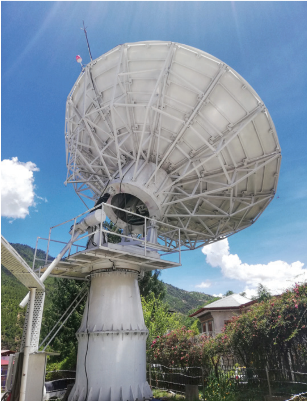
South Asia Satellite (SAS) Ground Station Antenna
